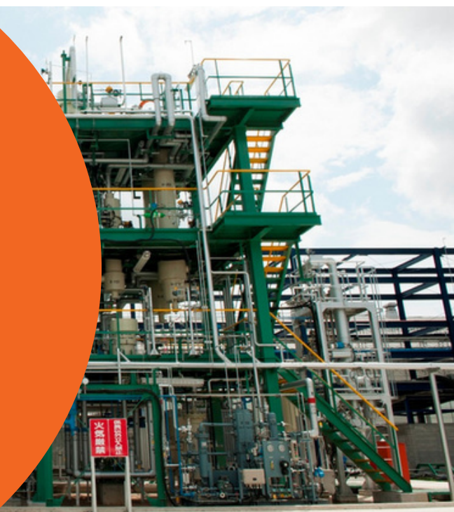
SPERA HYDROGEN® demo plant / Courtesy Chiyoda Corporation
